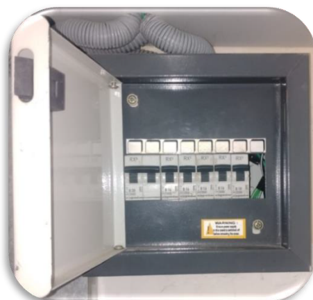
Figure 6.15: Miniature Circuit Breaker Switches
