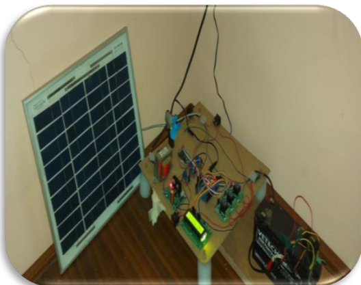
Implementation of Smart E-Vehicle Charging Station powered by Renewable Energy
