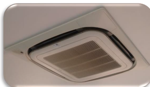
Figure 6.17: Air Conditioners in System Laboratories
